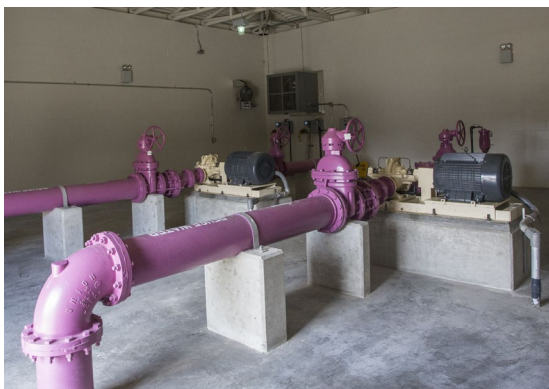
Purple Pipe to Distribute Reuse Water.
