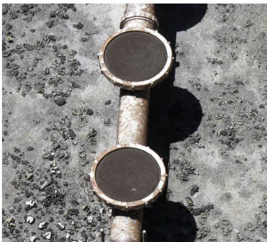
Fouled Diffusers Create Loss of Efficiency and High Energy Use.
