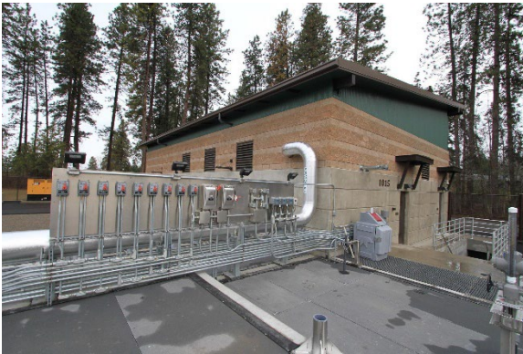
Coeur d'Alene Tertiary MBR with Chemical Sludge Aging. Reprinted with permission from HDR Engineering, Inc.
