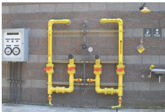
Chemical Receiving Station.
