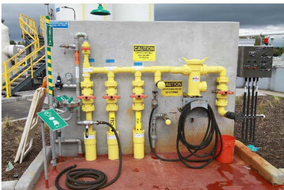
Chemical Dosing Station.
