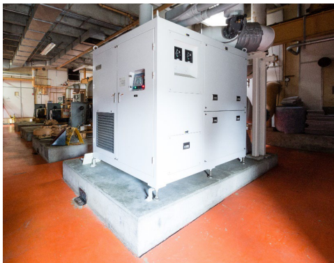
Blowers Are a Key Power-Consuming Process. Reprinted with permission from HDR Engineering, Inc.
