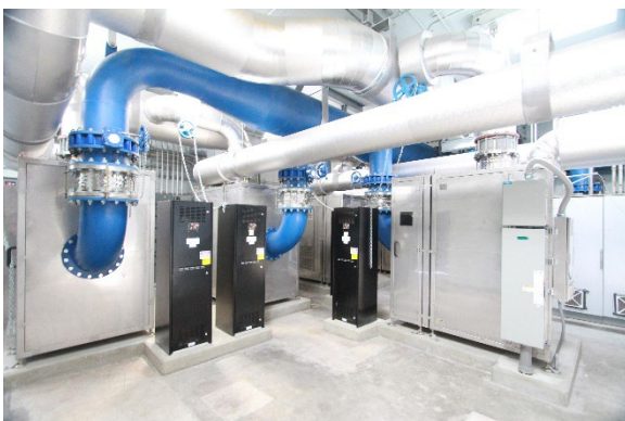
Blowers Are Key Energy-Consuming Equipment.
