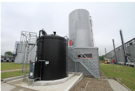
AirPrex Installation, Saltzitter, Germany.
