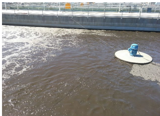
Unintended Aeration by Liquid from Aerobic Zone Returning into Unaerated Anoxic Zone.
