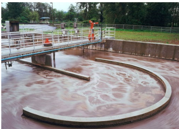
Simultaneous Nitrification and Denitrification Can Achieve TN Reduction.
