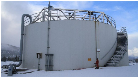
Primary Sludge Fermenter.
