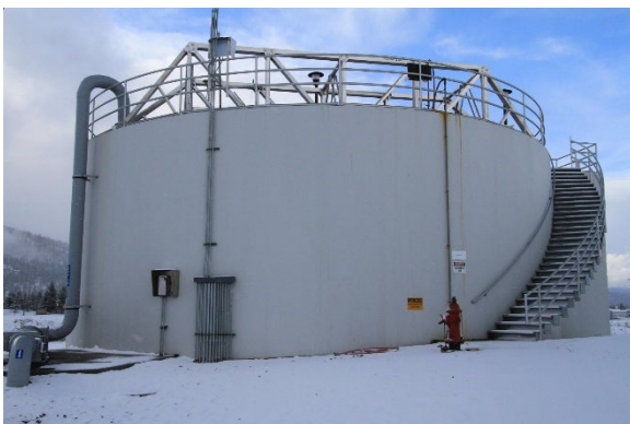
Primary Sludge Fermenter.
