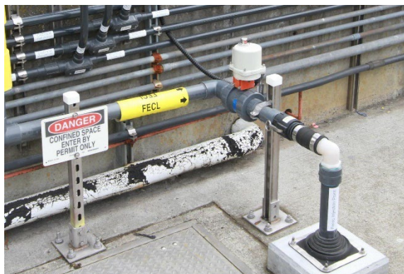
Ferric Injection Point.
