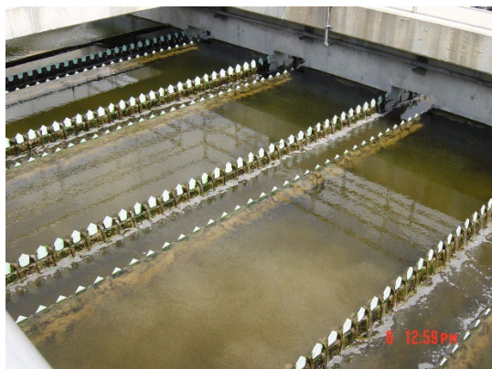
Performance of Two Parallel Secondary Clarifiers: without Baffle Modifications.
