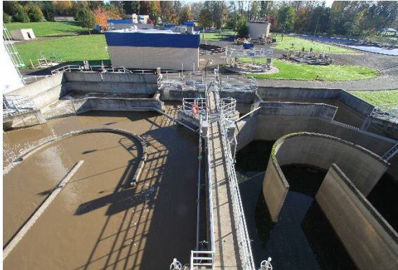
Simultaneous Nitrification and Denitrification Can Achieve TN Reduction.
