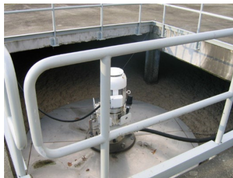
Covered Mechanical Sparger in Opened Basin to Aerate with Pure Oxygen Supplied under Cover (Linde).
