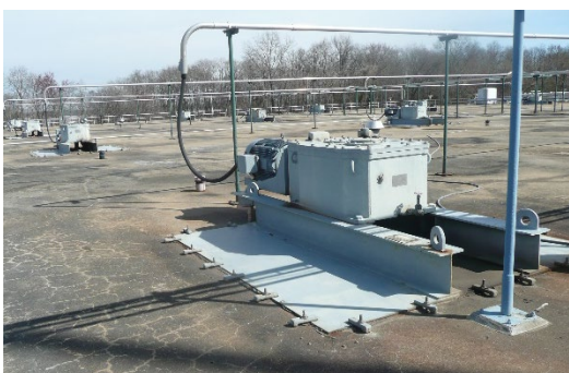
Typical Covered HPO Basin with Mechanical Mixers/Spargers for Aeration.
